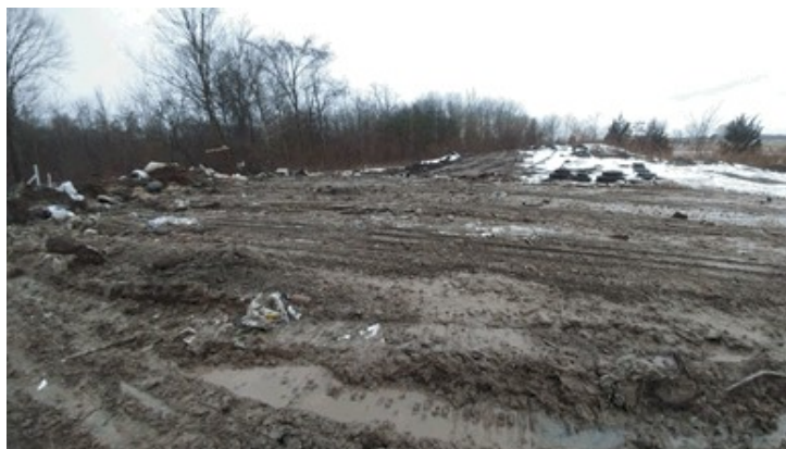
Active waste cell later that afternoon (pushed and covered). Picture taken and sent by Mr. Sholdice
